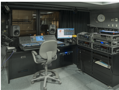
The audio control room at the Kani Public Arts Center small theater, featuring a Yamaha CL5 console
